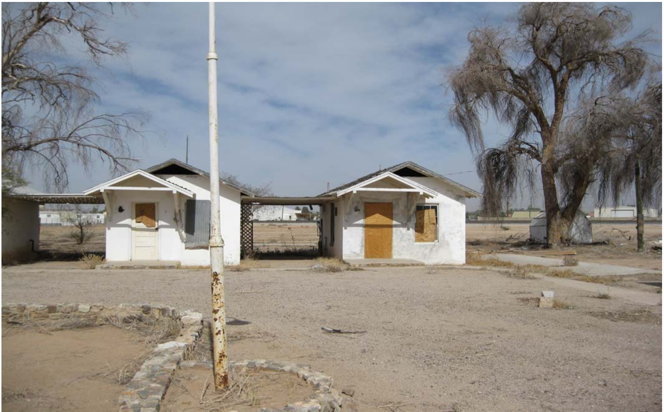
Courtyard with the 8 cabins (all vacant and in poor condition).
